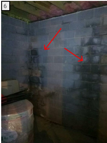
Correction needed before basement completion is performed
